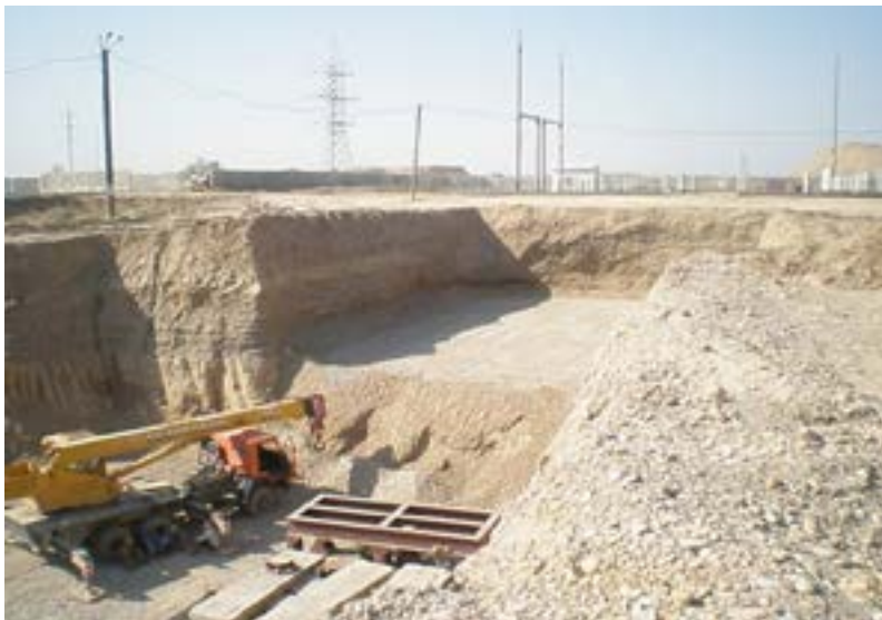
Figure 10. Terracing of a soil cushion at one of the workshops of the Standard-cement plant in South Kazakhstan region
