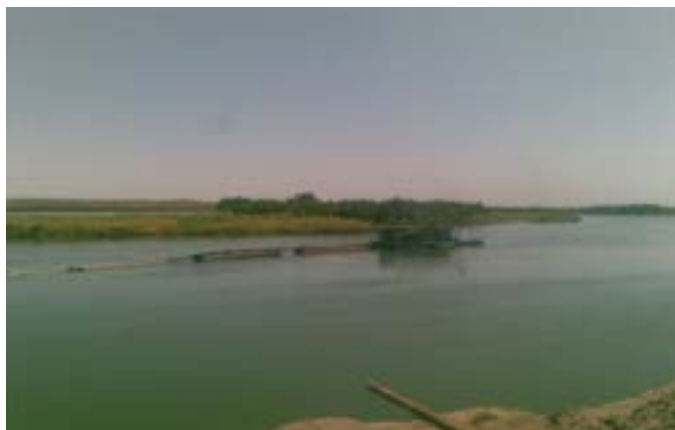
Figure 5. Pumping station on a floating pontoon
