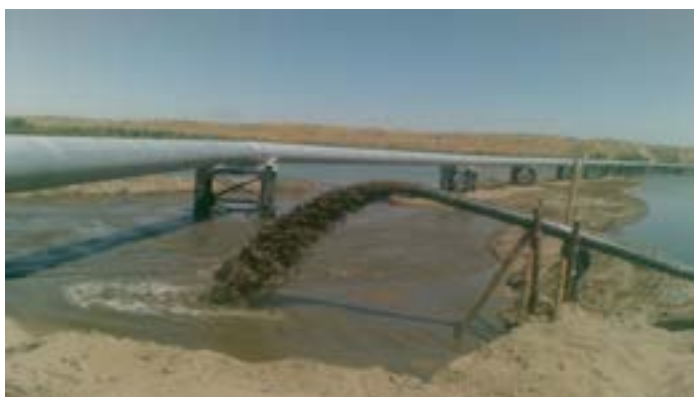
Figure 6. Formation of the body of a temporary dam using the alluvium method across the Syr Darya River in the Chardara region of the South Kazakhstan region
