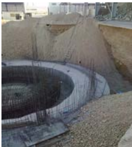
Figure 2. Device for backfilling soil into the cavities of the pit of a ring foundation at the Standard-cement plant in South Kazakhstan region
