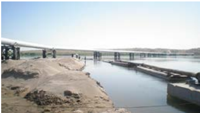
Figure 4. General view of the gas pipeline on metal supports
