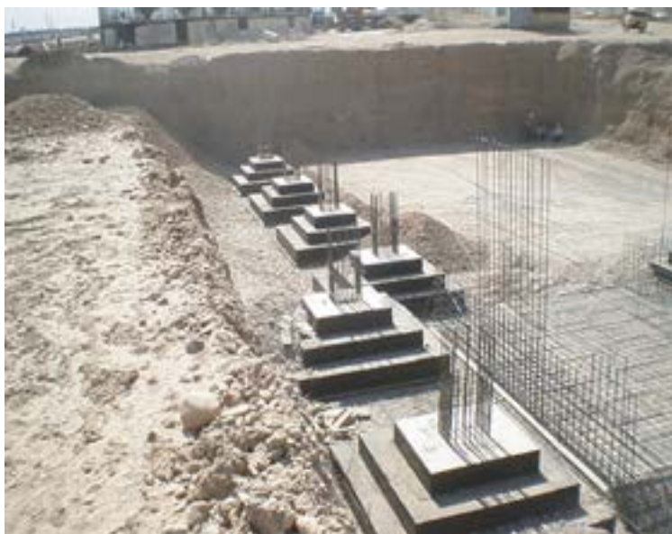
Figure. 11. Construction of shallow foundations on an artificial cushion of local gravel-sand soil in one of the pits of the South Kazakhstan region
